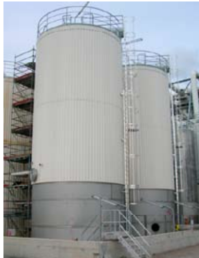
Ethanol storage tanks, BNEP, Lillebonne
