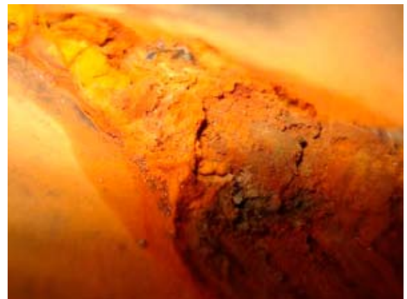
Untreated welded joint showing severe corrosion after only 1.5 years in operation
